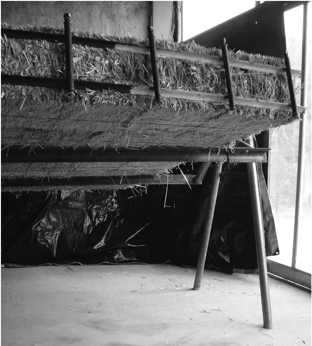
Fig. 24 The wall section is winched onto a special frame that enables the wall section to be rotated about a horizontal axis through the centreline of the wall. In this position it may be prime-plastered and then rolled into place after attachment to a relocation frame in the vertical orientation.
